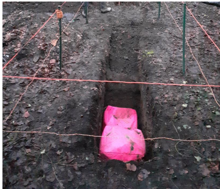
The ditch trench being dug out. The pink items are the fall arrest system
