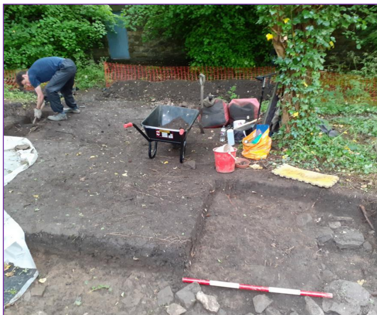
Work starting on the Saturday 19 th June, looking east towards the boundary wall
