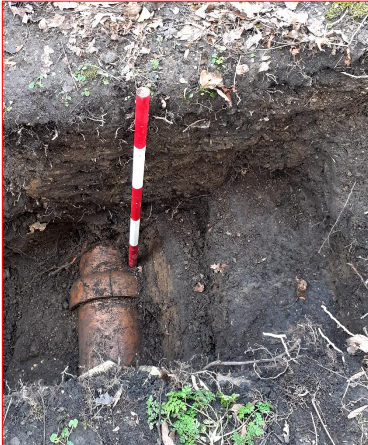
The “10 inch” ceramic pipe in the west end of the trench, looking south
